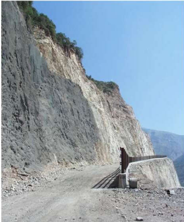
Careful blasting and the addition of a fence barrier to prevent rockfalls from bouncing onto the slope below.
