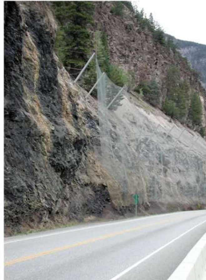
Light mesh draped on a slope to prevent small rockfalls from bouncing outwards.
