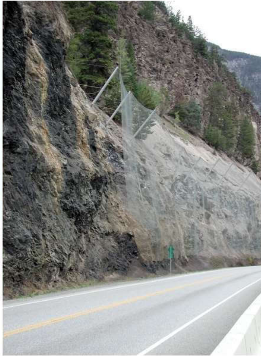
Light mesh draped on a slope to prevent small rockfalls from bouncing outwards.
