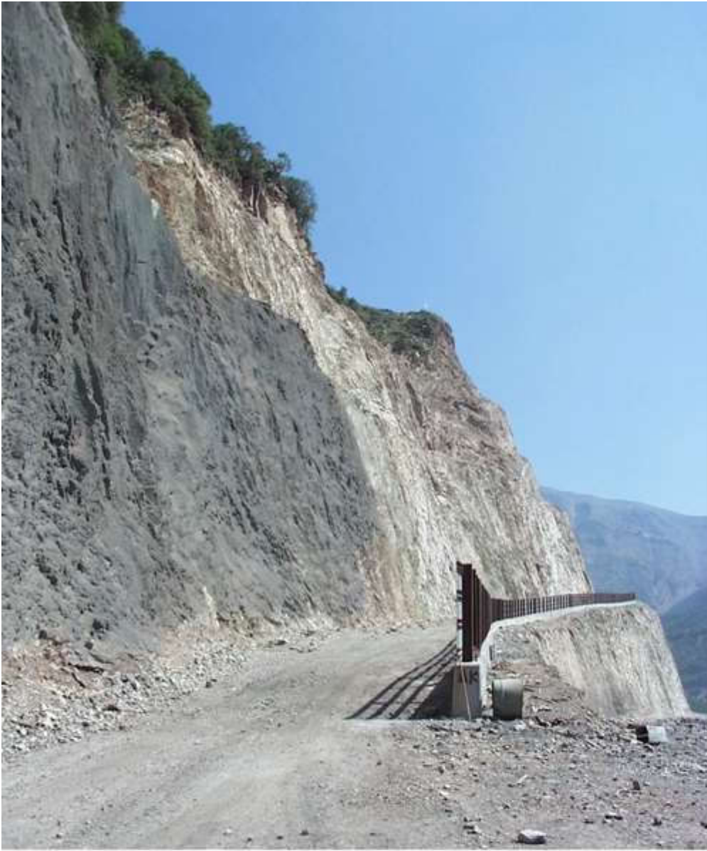
Careful blasting and the addition of a fence barrier to prevent rockfalls from bouncing onto the slope below.
