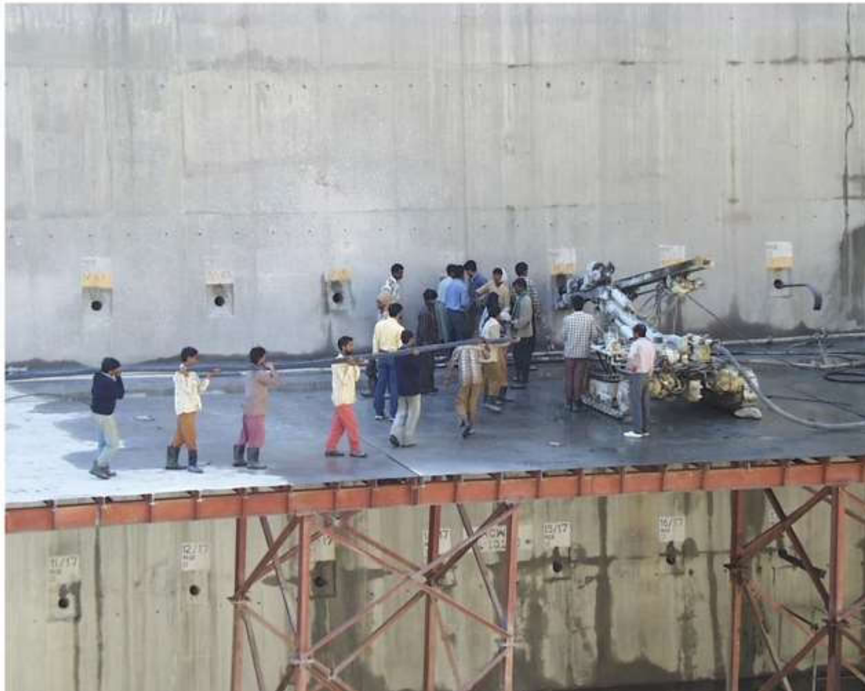
Drilling long holes for cables and installing a cable in a concrete buttress.
