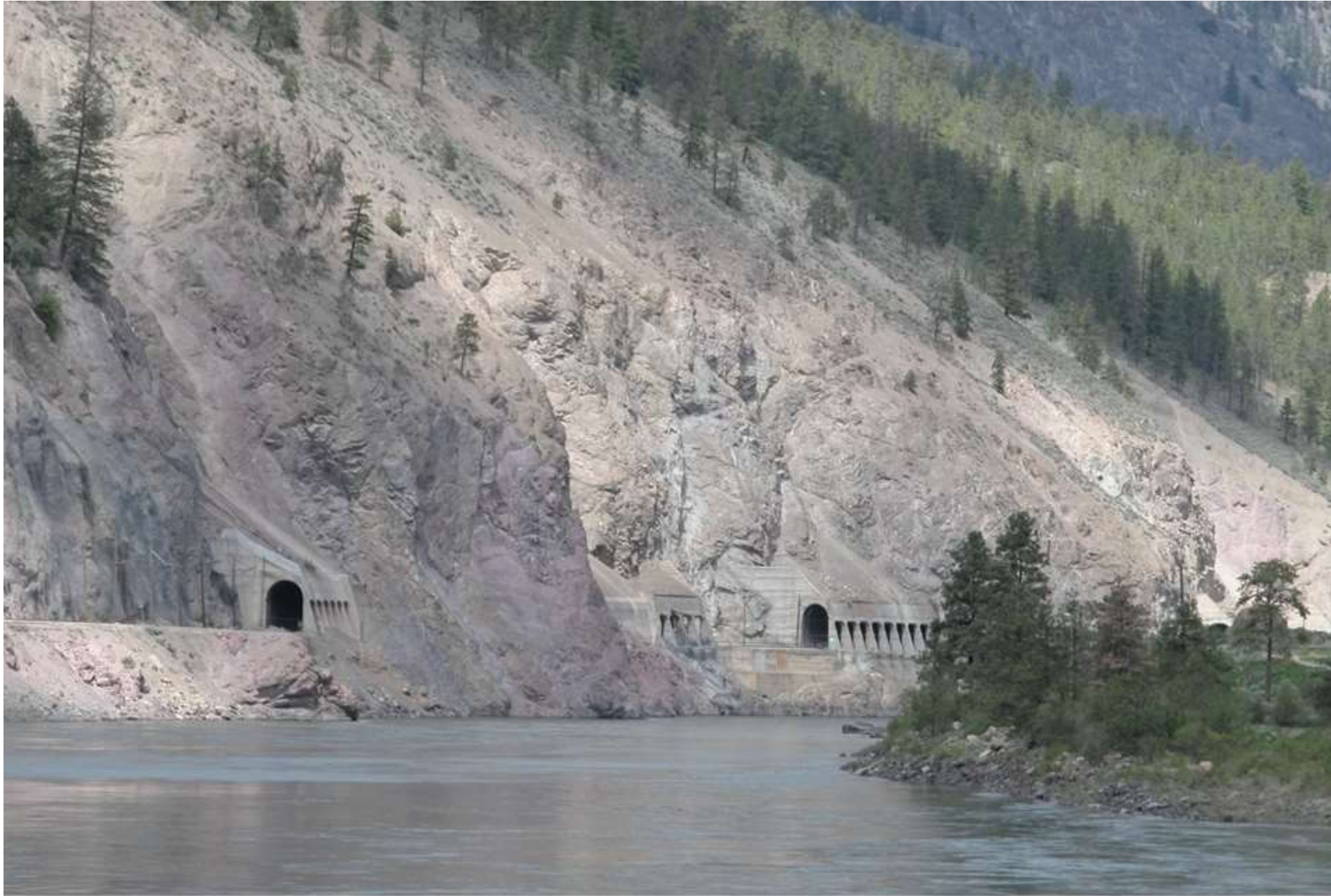
Rockfall and avalanche shelters over a railway line at the toe of a steep mountain slope.
