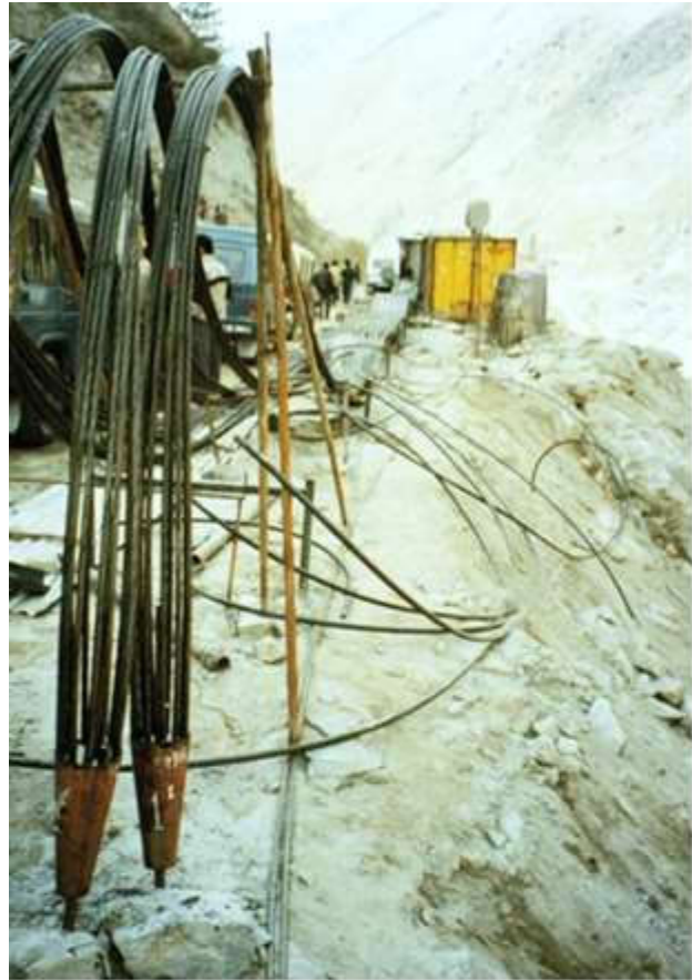
Long high capacity cable anchors prepared for installation in a concrete buttress at a slope toe.
